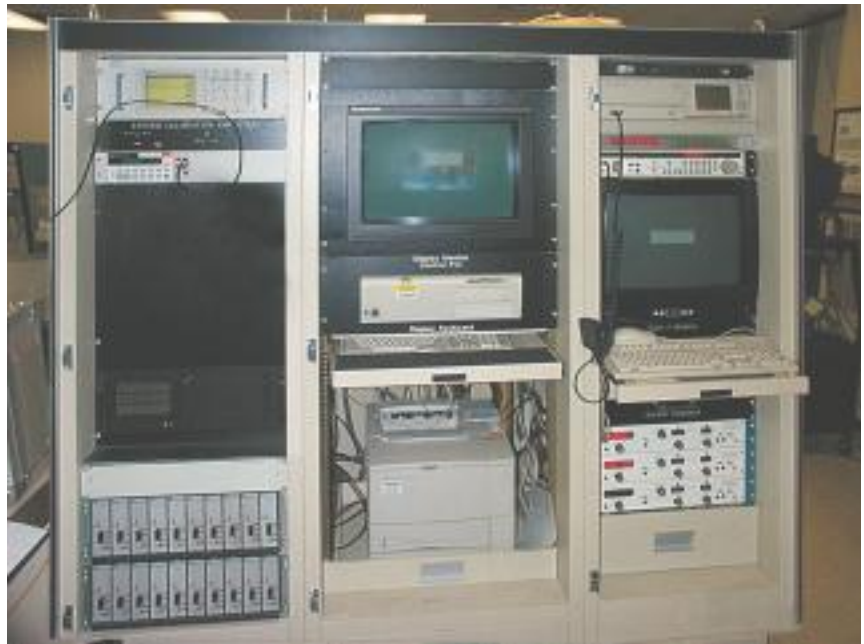
Figure 1. The Pratt & Whitney Rotating Machinery Analysis System. The VME cage is accessible from the rear of the rack. (Courtesy of Pratt & Whitney)
