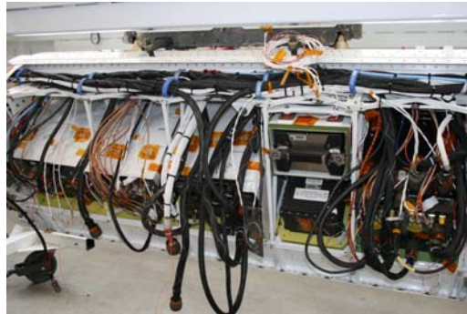
Figure 3. Photograph of the UAVSAR with the cover removed shows how the electrical subsystems are arranged within the pod. (Photo courtesy of JPL)
